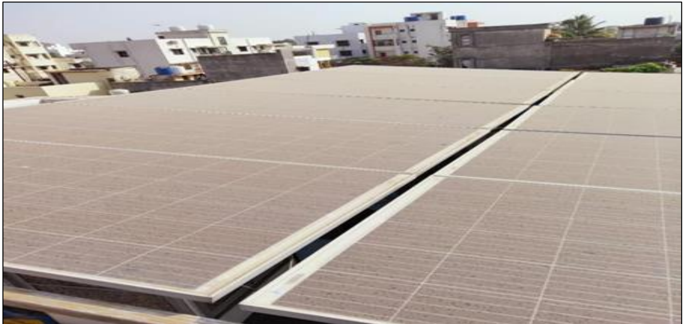
Fig 1 Solar Panel Problem
